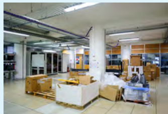
Setup of the technical room for 4-FLIGHT at Marseille ACC.
