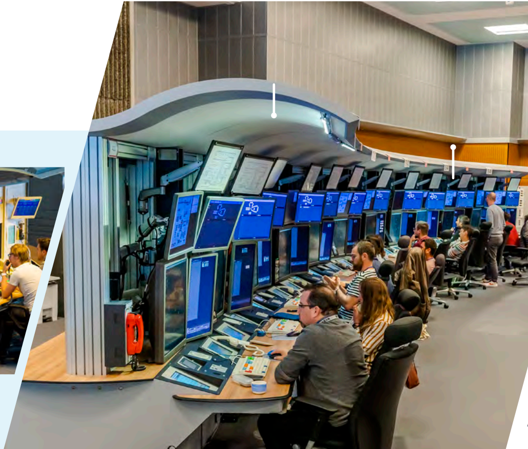
...to the 4-FLIGHT/Coflight system (on June 14, 2022 4-FLIGHT was officially declared in service in Reims ACC — a first for DSNA!)
