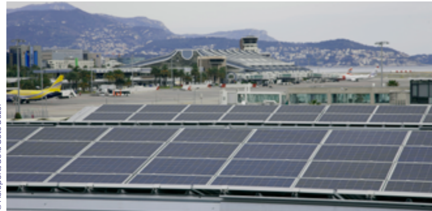
Solar panel-covered car parks, Nice airport
